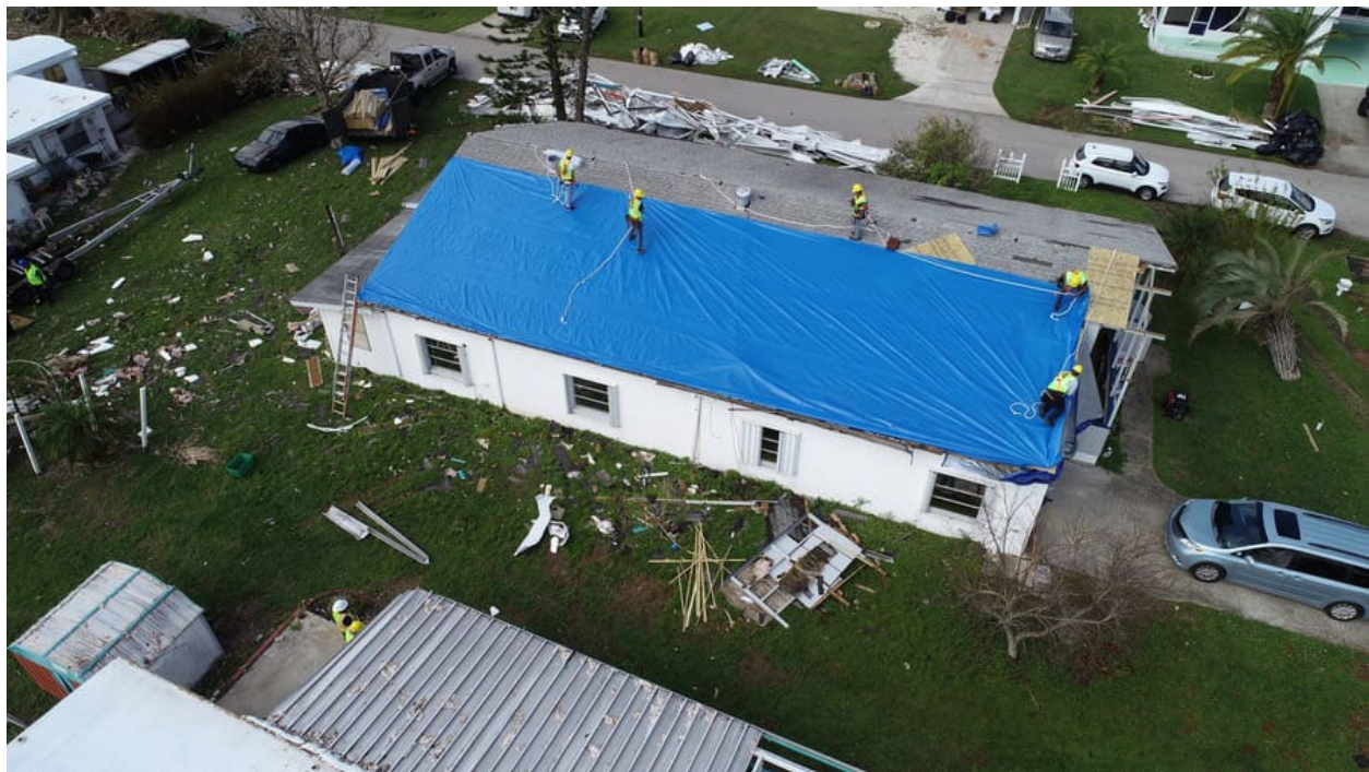
Figure 1-4. Hurricane Ian Housing Damage in Sarasota County 5
