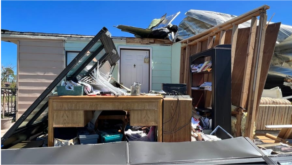
Figure 1-2. Hurricane Ian Damage in Sarasota County 3
