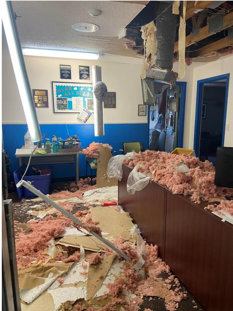
Figure 1-6. Hurricane Ian Interior Damage to the Boys & Girls Club in City of North Port 7
