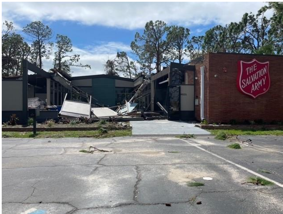
Figure 1-5. Hurricane Ian Damage to the Salvation Army of Sarasota County North Port Facility 6
