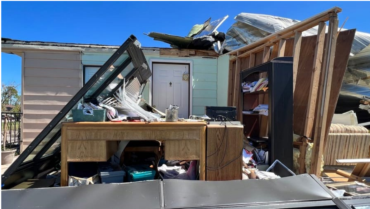
Figure 1-2. Hurricane Ian Damage in Sarasota County 3
