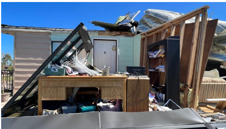
Figure 2: Hurricane damage to manufactured home
