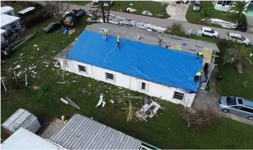
Figure 5: Hurricane Ian Housing Damage in Sarasota County
