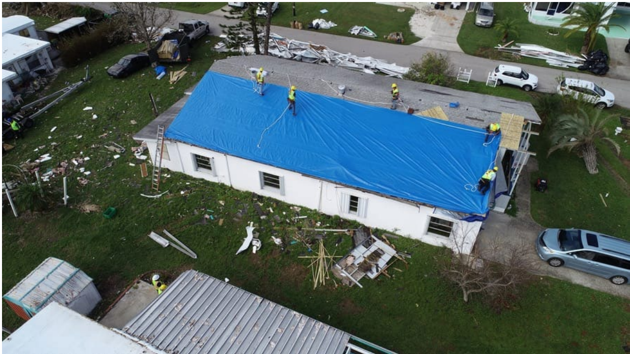
Figure 1-4. Hurricane Ian Housing Damage in Sarasota County 5
