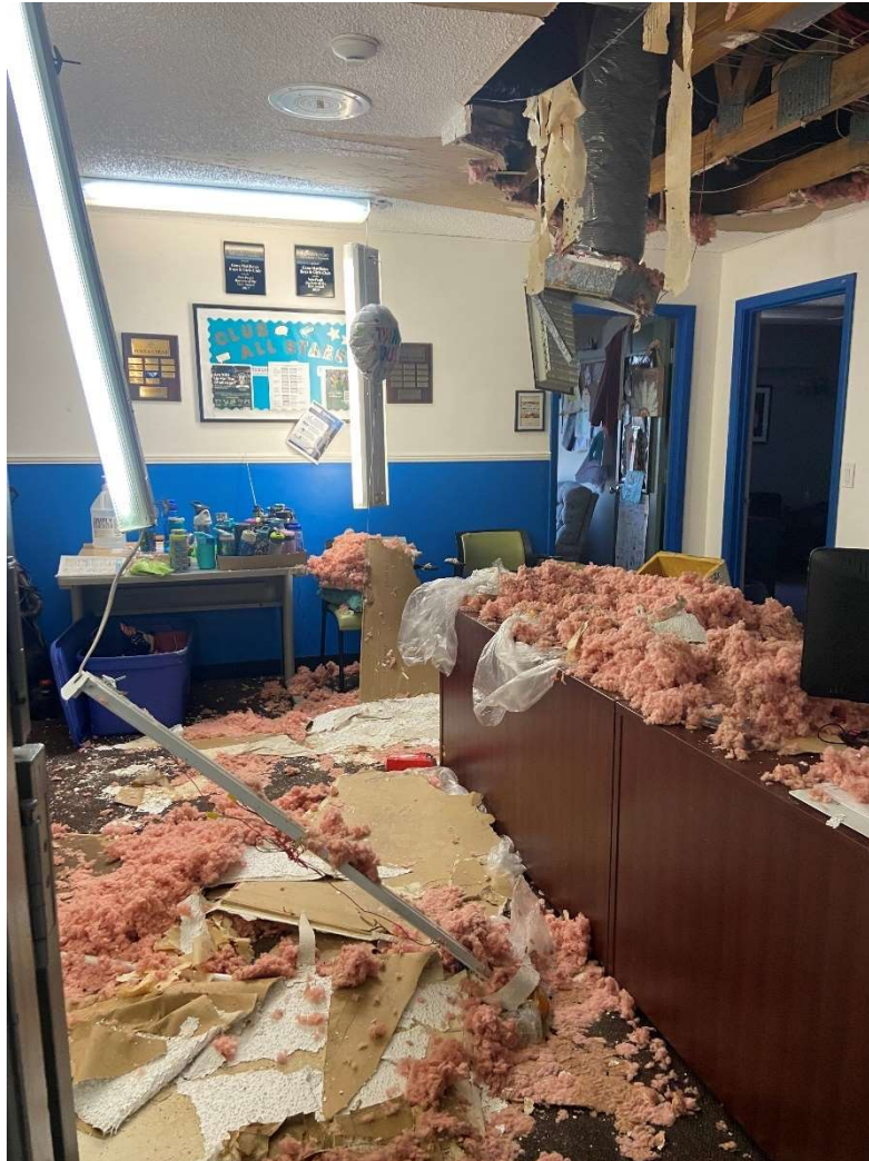
Figure 1-6. Hurricane Ian Interior Damage to the Boys & Girls Club in City of North Port 7
