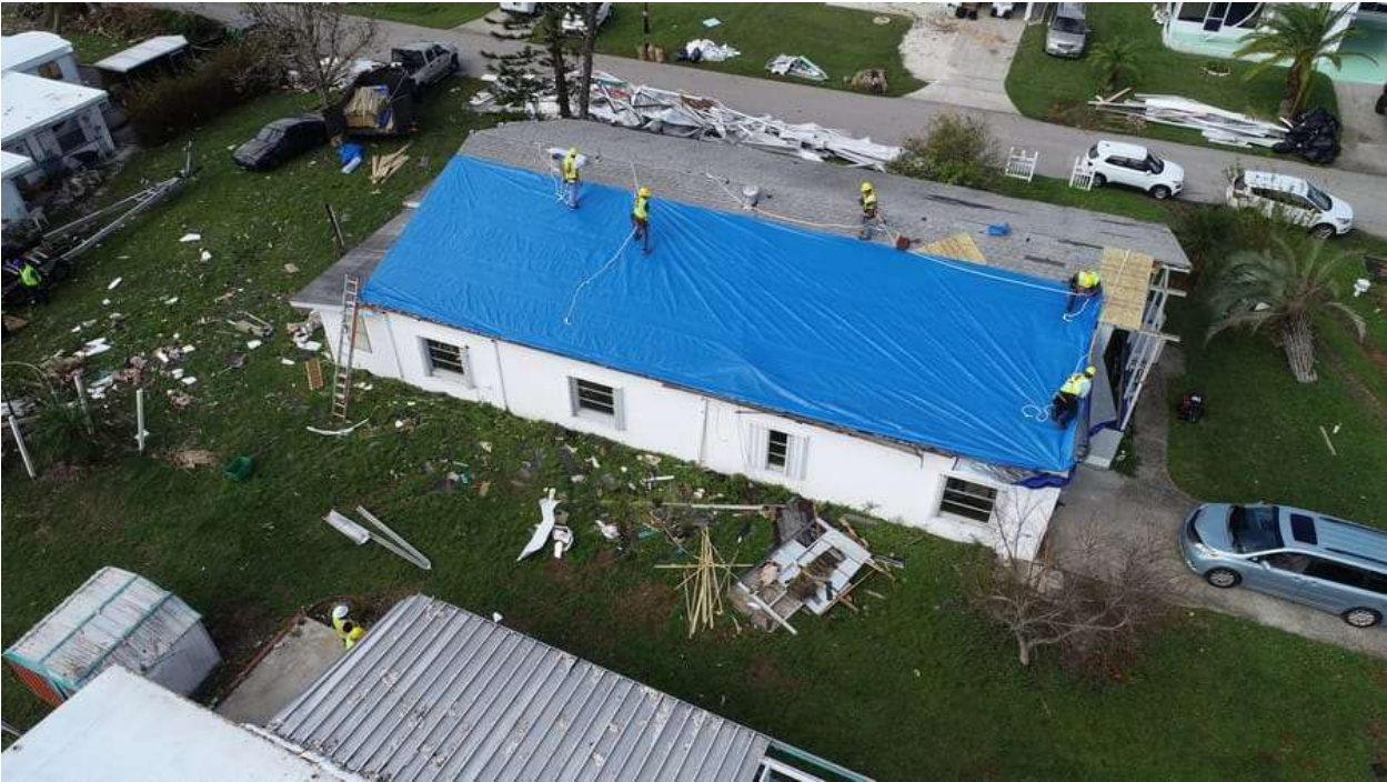
Figure 1-4. Hurricane Ian Housing Damage in Sarasota County 5
